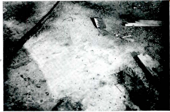
Flat Scaling Caused by Concrete Surface Freezing Before Coverage was Applied. The Defect did not Affect the Structural Quality of the Slab
