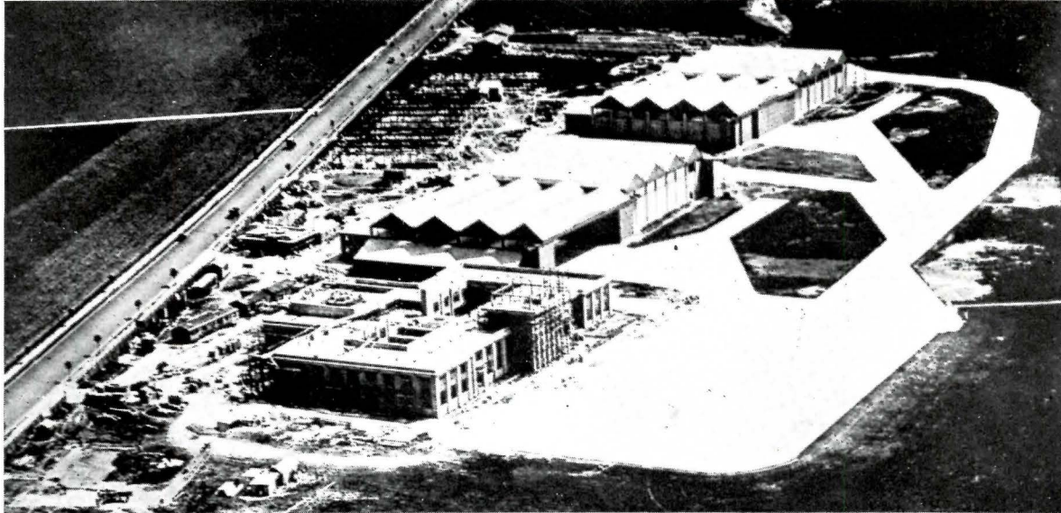
Construction in Progress, New Croydon Airport with System of Concrete Aprons and Maneuvering Space
