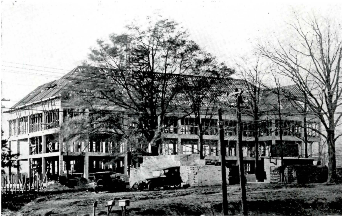
Reinforced Concrete Frame of Building Shown on Opposite Page Hentz, Reid & Adler, Architects
