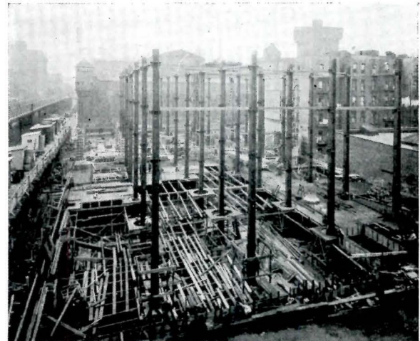
Framing of the Uppercu-Cadillac Building. The Floor Construction is of the Girderless Type Charles E. Birge, Architect
