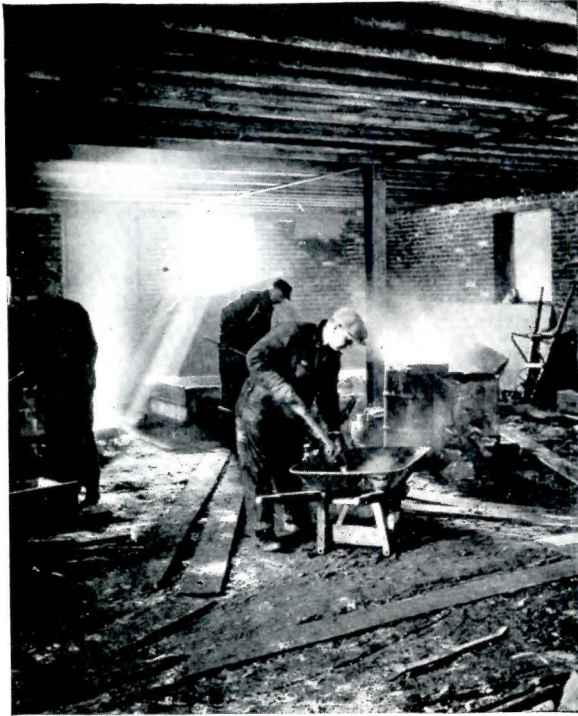
Interior Brickwork and Proper Temperature Control. Note Muslin Covering Door and Window Spaces, and Salamander Placed to Effect Equal Radiation of Warmth
