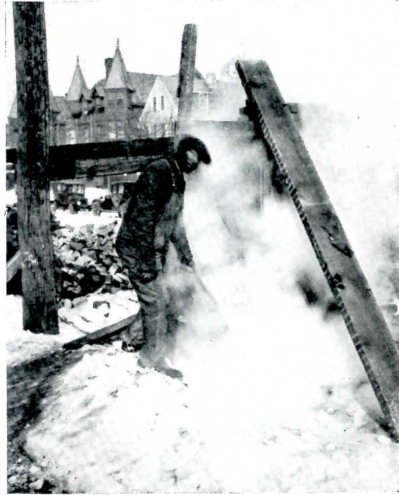
Thawing Out a Snow-covered Pile of Bricks with Steam Hose Should not be Necessary. Brick Should be Stacked with Complete Coverage of Top and Sides of Stack
