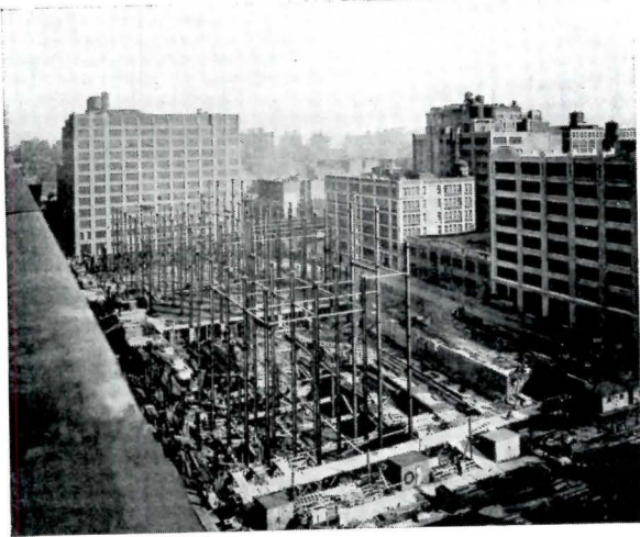
Framework U. S. Appraisers' Stores, Combined Long Column-cores with Girderless Floor System
