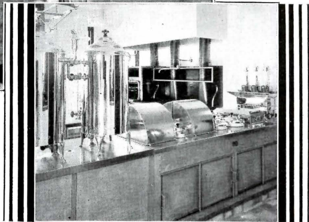
Those who use and those who specify equipment invariably prefer Van products—because of low cost, negligible upkeep and long life. Shown here is part of a recent Van Kitchen in the Christian B. Holmes Hospital, Cincinnati, Ohio.
