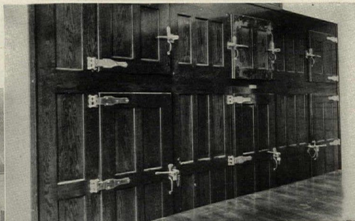
A small part of the 20,000 cubic feet of "Lorillard" refrigerators, installed by Van for use in connection with the West Point kitchens, bakery and mess halls.
