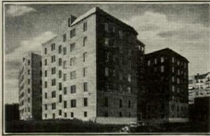
37,000 sq. yds. of the new RIBBED STEELTEX safeguard walls and ceilings in this outstandingly beautiful modern apartment building, The Grenfell, now under construction at Kew Gardens, L. I., N. Y. Economy of construction, adaptability, and tenant satisfaction, no upkeep costs—influenced the Gormac Construction Corp., Brooklyn, N. Y., owners and builders, to build with reinforced plaster.
