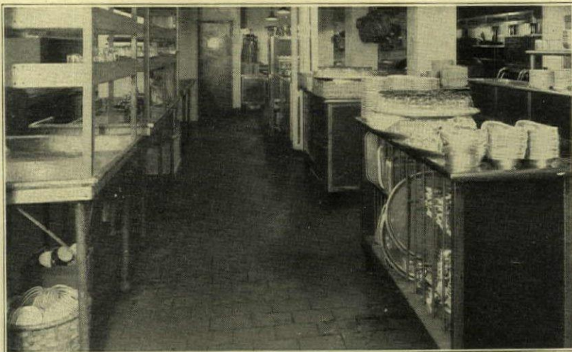
The compact kitchens for the Governor Clinton Grill and Coffee Shop. The dishwashing section is at the left; in the background is the range and broiler division.
