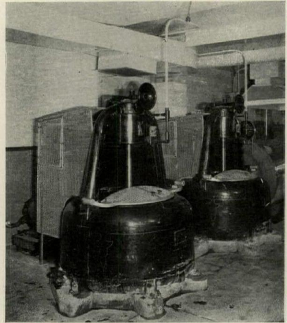
Extractors Should Be Securely Anchored to the Floor
