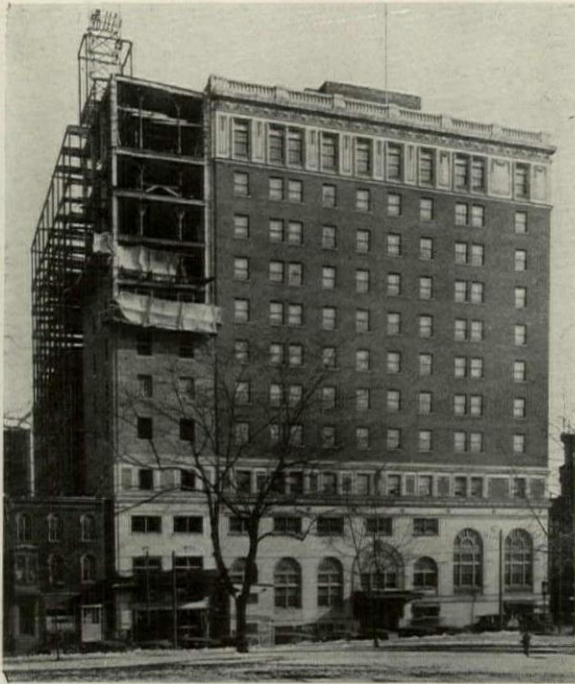
Addition to Hotel Not Originally Designed for Additions. Property Acquired Later. Penn Harris Hotel, Harrisburg
