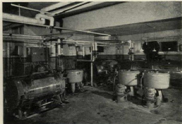
Extractors and Washers Should Be in Close Proximity for Efficient Operation
