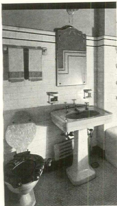
Bathroom in Eddystone Homes, 401 Melrose Street, Chicago, Ill., showing STANDISH vitreous china lavatory with Kohler Dynamic combination fittings. VICEROY bath is equipped with Rapidrain. Architects, Holabird & Root; General Contractors, A. W. S. Construction Co.; Plumber, Charles R. Ewing, Jr.; Jobber, Western Plumbing Supply Co.
