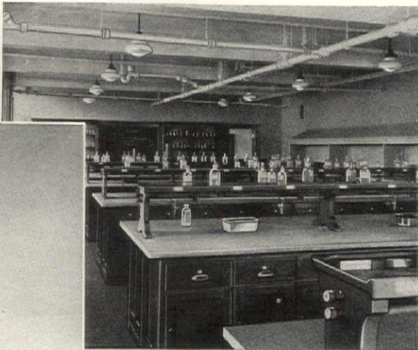
One of the laboratories, showing Duriron drain piping hung from the ceiling.
