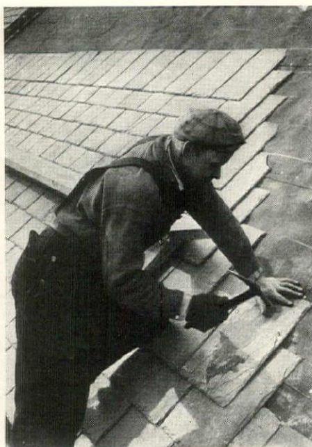
Ebenezer Community Building, Chicago, showing how slate is nailed directly to the roof-deck of Federal Nailing Concrete Slabs. Archt., Andrew E. Norman.
