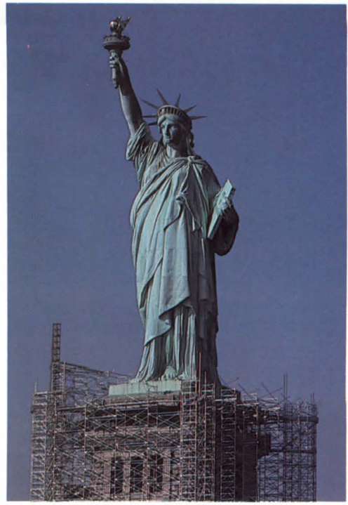
Recent photograph of the Statue of Liberty with its partially dismantled aluminum scaffolding system.
