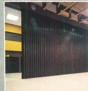
Code Required Area Separation preserves the design prerogative for large open space areas.
