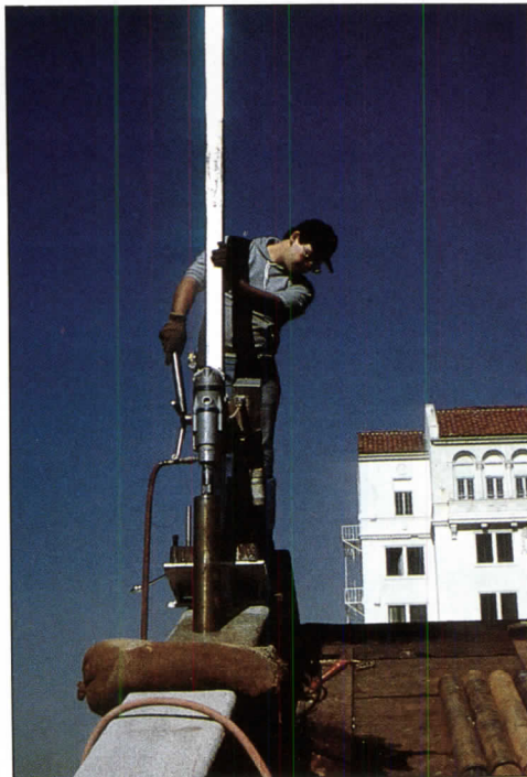
Workers core a masonry wall prior to placing and grouting rebar for seismic compliance.
