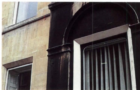
This limestone building in Bath, England, shows the effects of plain water cleaning on years of accumulated soot and grime.
