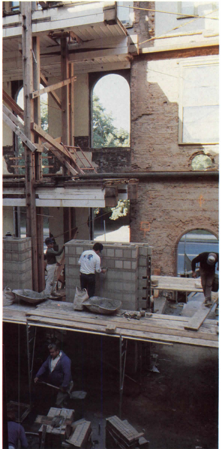
Right, workers construct a new masonry structure within the shell of the old building, with stabilizing structure above.
