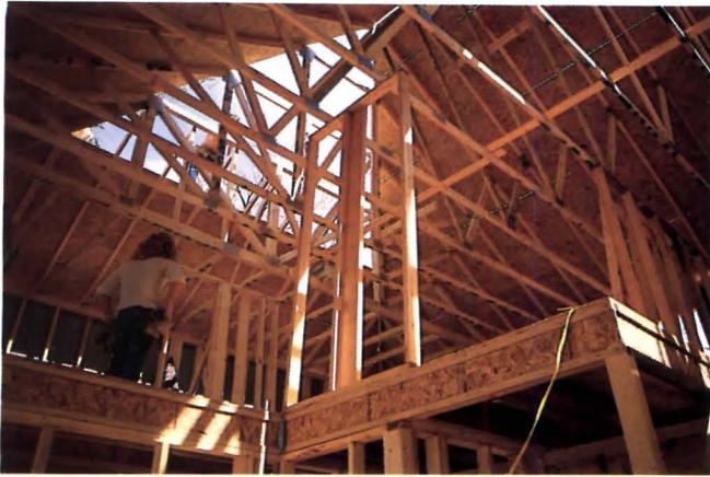
Above, an effective system of automated mass-produced housing is alive and well in America. It is based on mass-produced components fastened with nailing plates and delivered on specially designed trailers large enough to hold an entire house that can be assembled in a single day (below).
