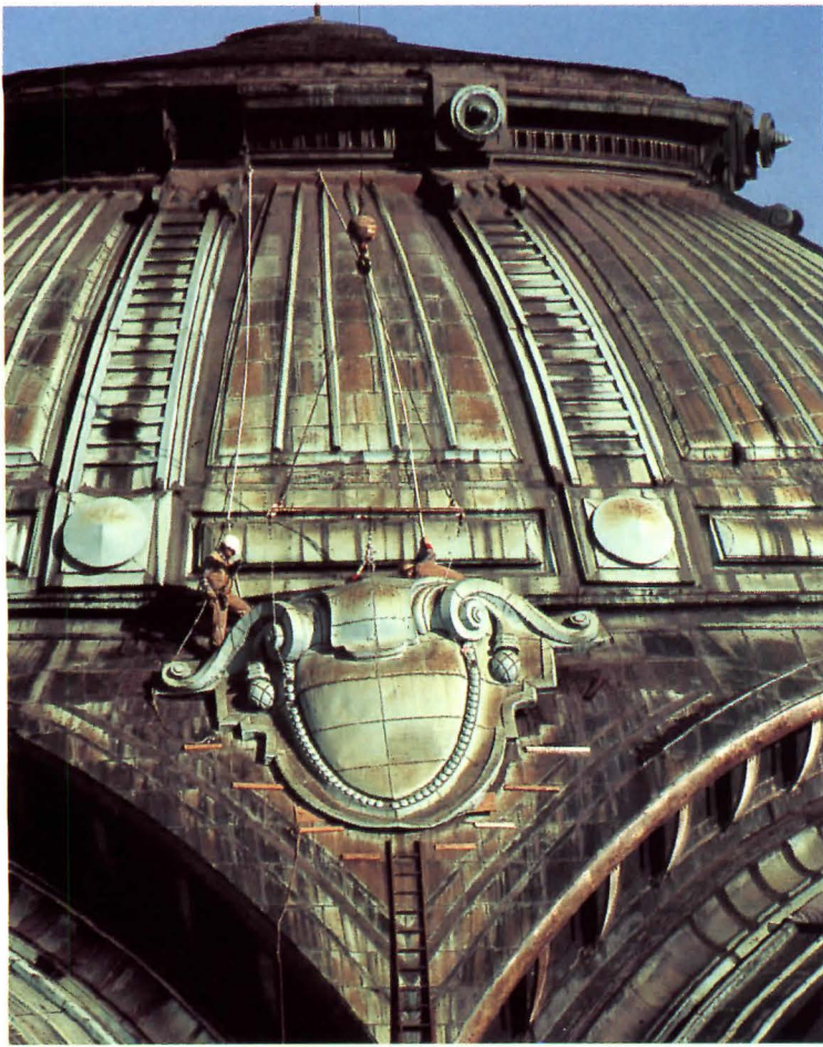
Left, an original cartouche, constructed of 16-ounce copper, crimped to improve its rigidity.
