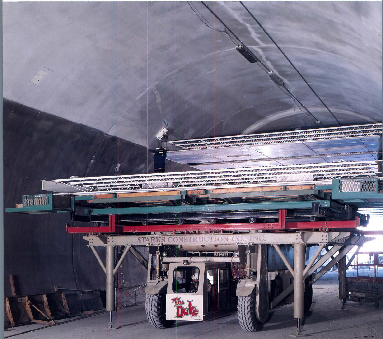
The "Duke" installing ceiling panels in the Hanging Lakes Tunnel, Glenwood Canyon, Colorado.
