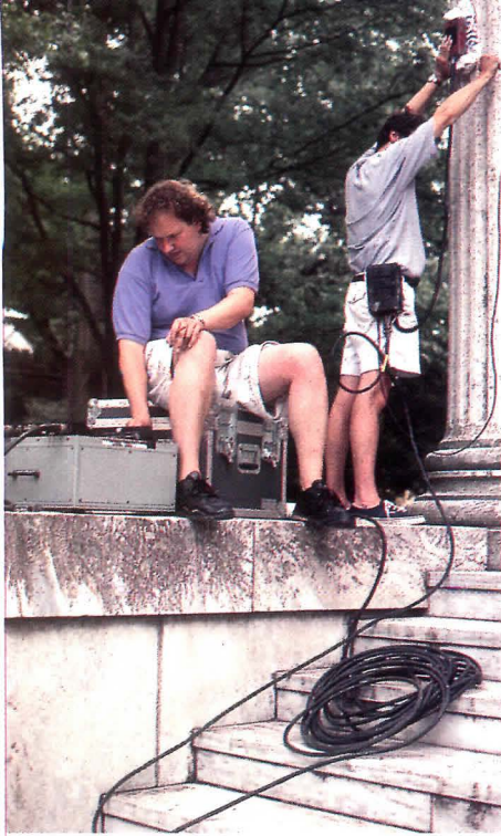
Engineers from G.B. Geotechnics survey lower portion of cracked marble column with hand-held radar.
