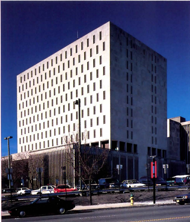
Limestone cladding of Essex County New Courts Building and Jail was one accident away from catastrophic failure. More than 20,000 Cintec anchors now prevent masonry's collapse.
