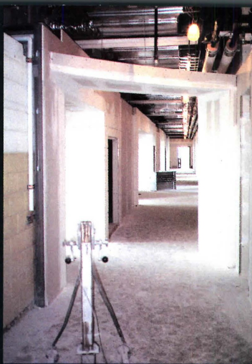
Architect gutted most interior spaces (above) during Colden Hall renovation, widened hallways, inserted "conversational" areas, and repaneled with gypsum board to provide clean, academic look that withstands abuse of high student traffic. Wall system also permits easy access to mechanical systems.
