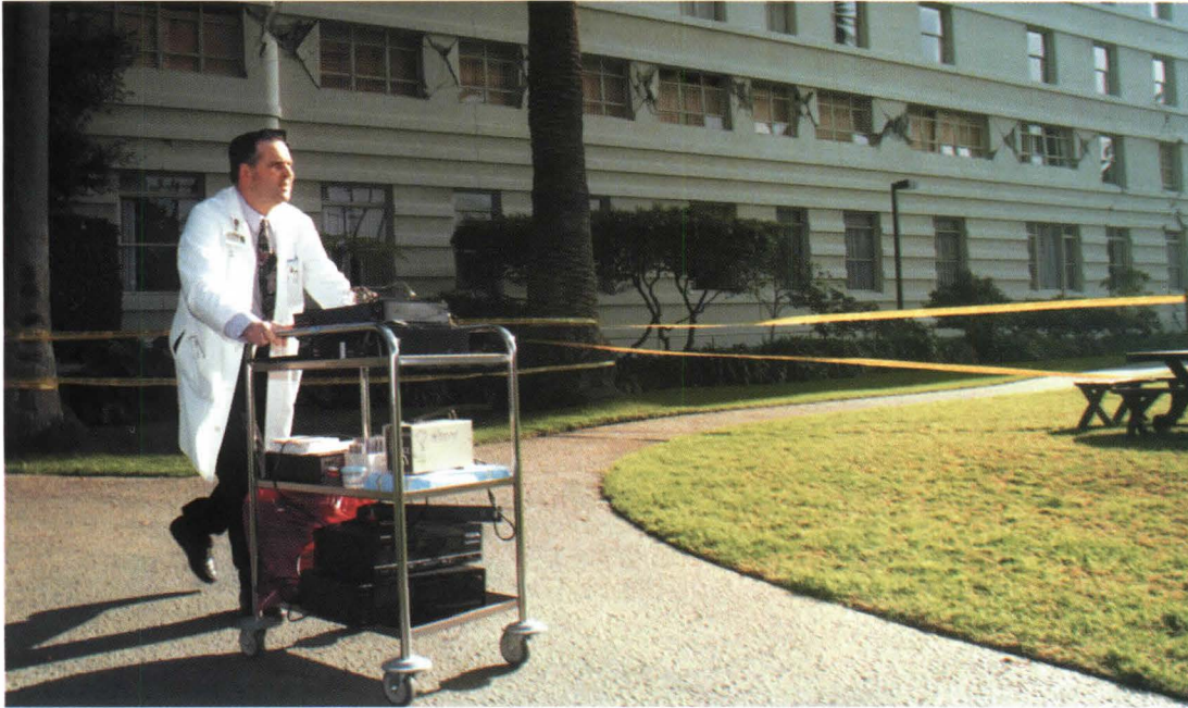
California lawmakers want to prevent earthquake damage, like this along the windows of St. John's Medical Center in Santa Monica.
