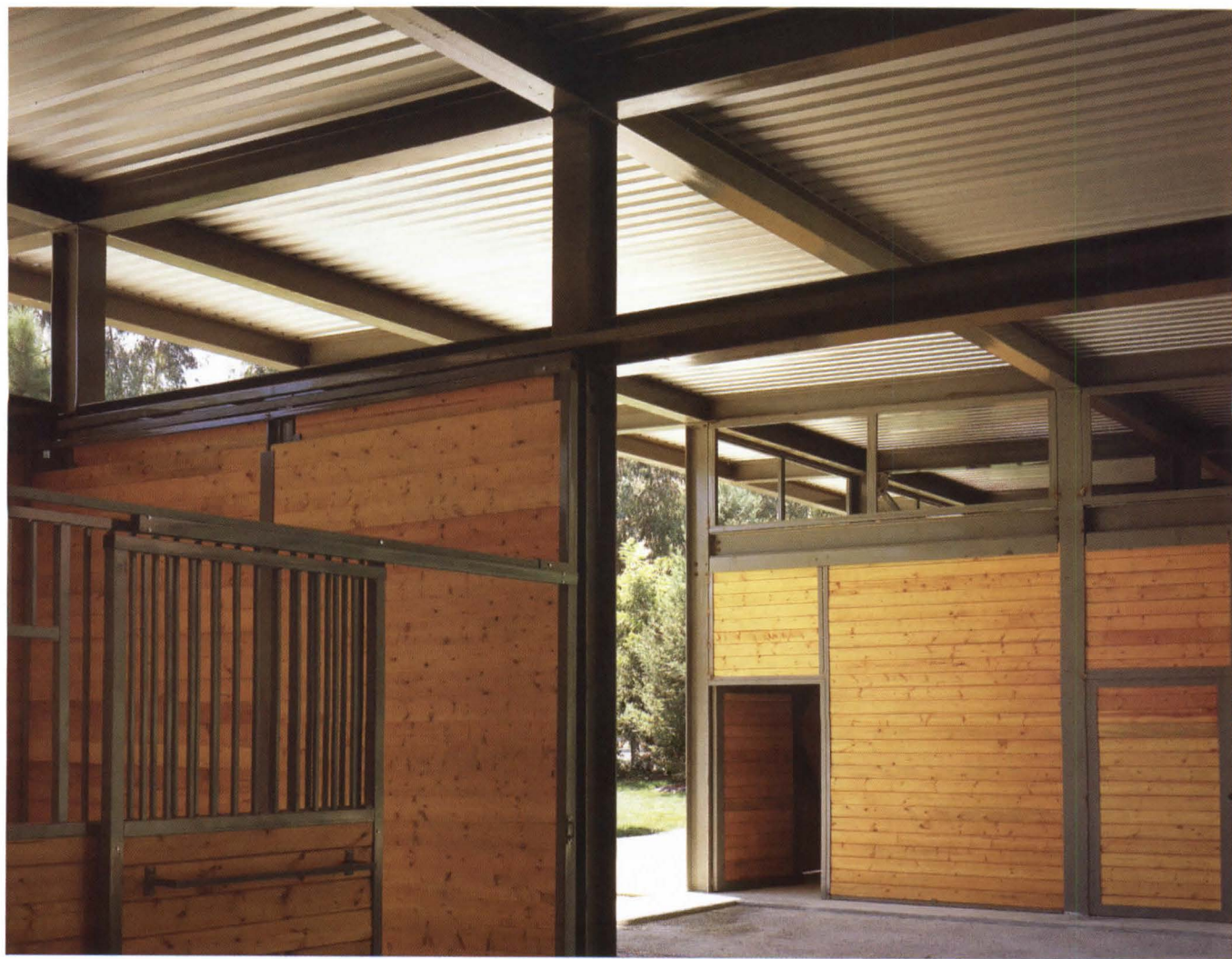
A 12-foot grid defines the structural system. The storage room (through door at right in photo) has a glazed clerestory, while the rest of the barn is open at the roof to ventilate the interior.
