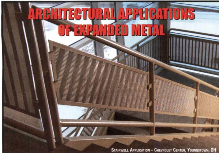
STAIRWELL APPLICATION - CHEVROLET CENTER, YOUNGSTOWN, OH
