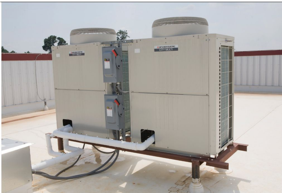
Rooftop System: The outdoor compressor units operate quietly and out of sight, skillfully directing cooling and heating refrigerant to 39 indoor fan coils.
