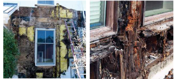
Water damaged walls.
