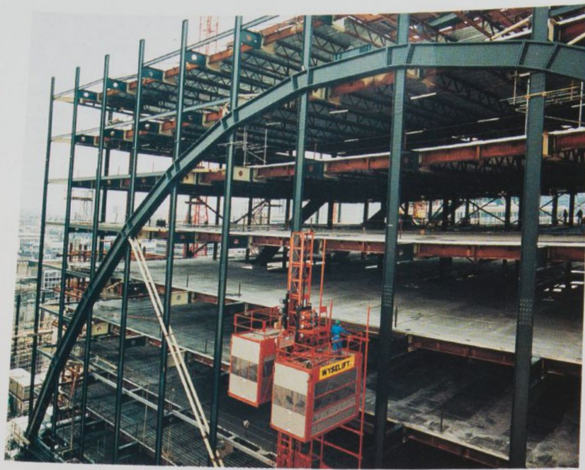
Floor trusses span the bays within the building and connect either to girders or directly to the exterior columns. The arches are constructed of parallel steel channels (above) with an intermediate space to allow the columns to pass through the arch (facing page, top left).
