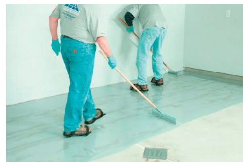
Polyaspartic coatings are typically used where there is fast return to service time desired, as they cure very quickly. Photo Courtesy of Bayer MaterialScience
