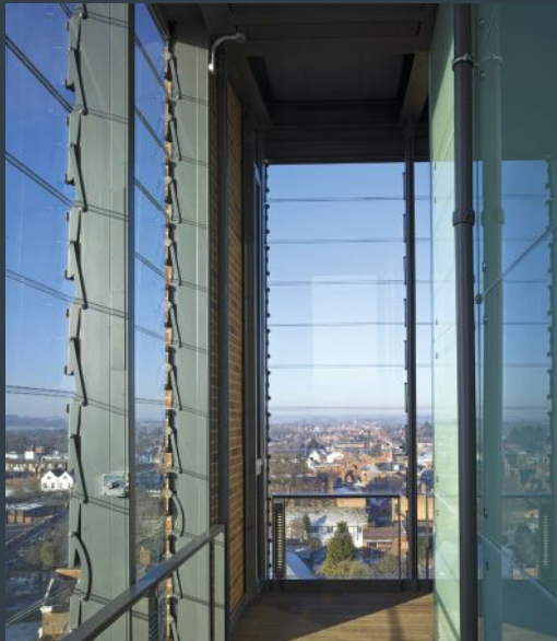
Louvered Facade Ventilators
