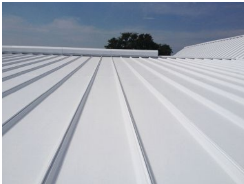
Reflective coatings are often applied over darker colored or aged reflective existing roofs to help reduce energy costs.
