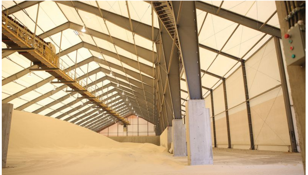
Figure 2 Source Energy Services: Inside a frac sand storage structure. Modern fabric buildings are allowing for a wide range of new and interesting designs.
