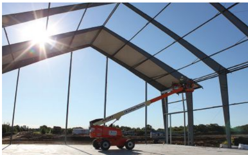
Figure 3 Rigid Steel Frame Structure: Fabric roof panels being kedered to a rigid frame building.
