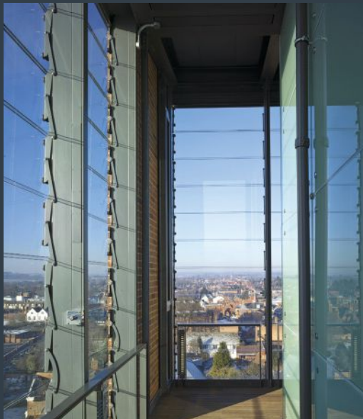
Louvered Facade Ventilators
