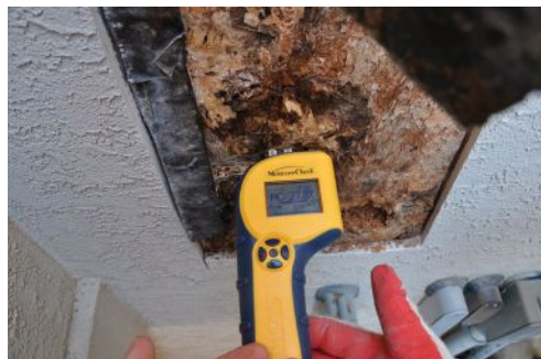
Most moisture problems are caused by poor architectural design that traps or directs water back into wall assemblies and does not allow sufficient drainage.
