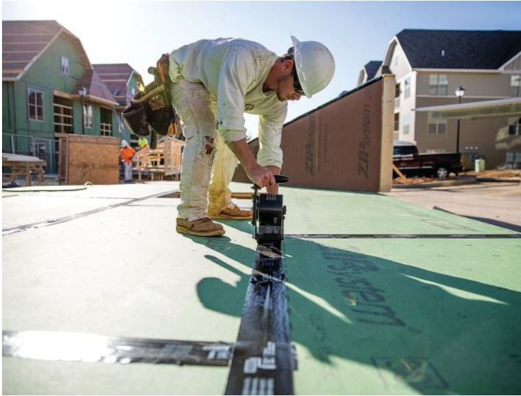
Installers pre-assembled ZIP System® sheathing panels and tape before installing on exterior walls and roofs.
