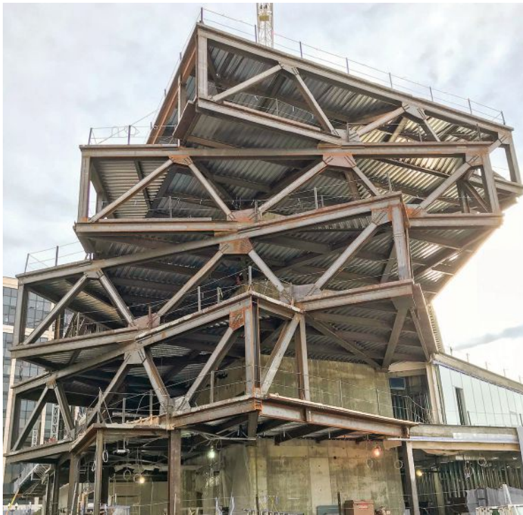
Structural steel framing for The Heights Building in Washington, D.C. Photo Courtesy of Silman/Gilbane
