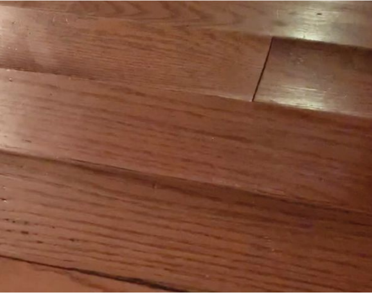
Trapped moisture due to vapor drive could damage both finish floor coverings and the subfloor below.
