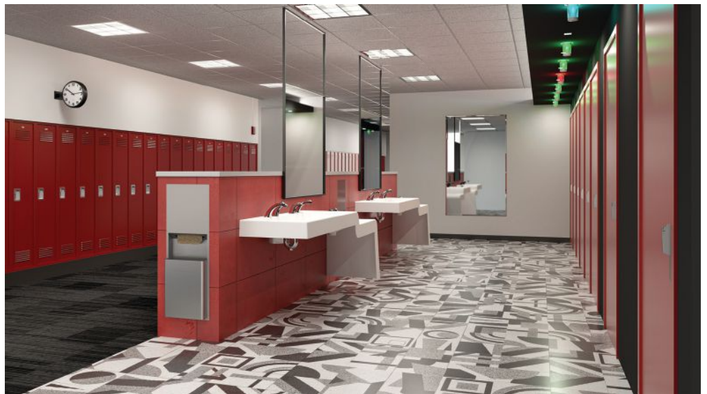
In schools and hospitals, sensor-operated fixtures are a highly effective way to reduce the spread of germs and bacteria because hand contact is not required for their use, and they greatly decrease instances of cross contamination resulting from multiple people handling infected fixtures.
