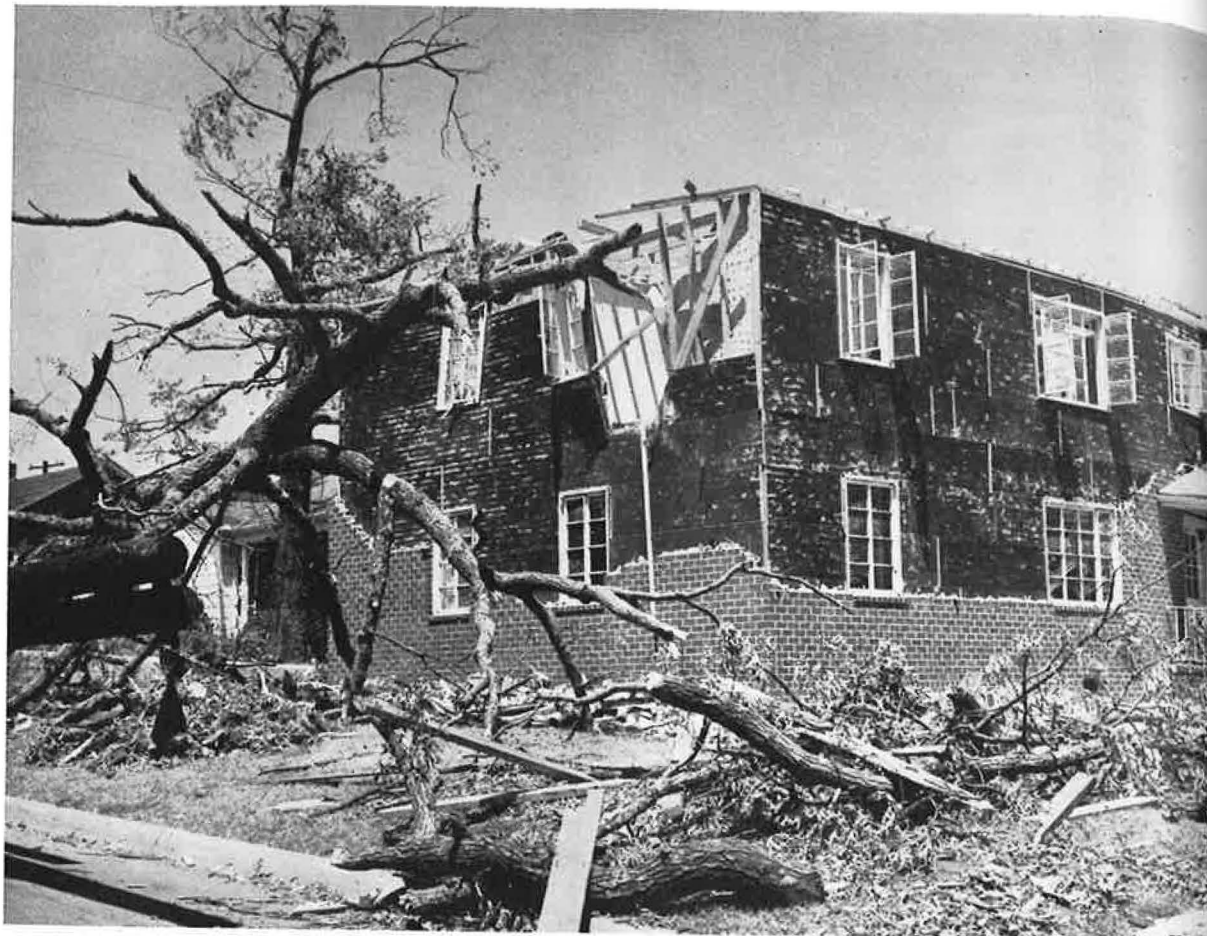
Roof and brick veneer inadequately anchored (Georgia)
