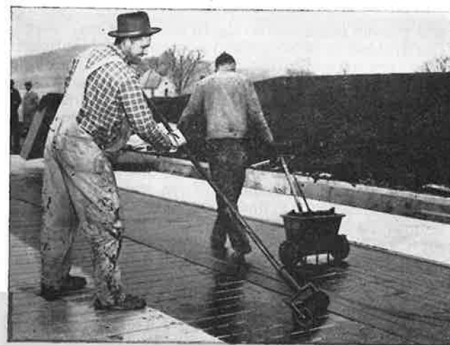
Semi-mechanical method for small jobs. Apply ribbons of adhesive with the Lexsuco Spreader, spread with roller coater and unroll vapor barrier into adhesive. Next, imbed insulation into ribbons of adhesive on top of vapor barrier.
