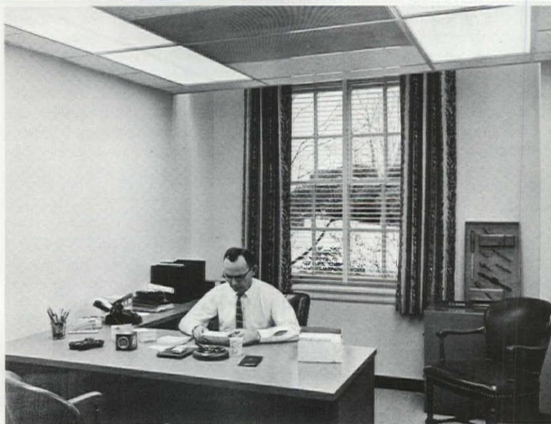
Floating panel luminaire in corner office (top) uses high-output lamps. Typical two-window office (bottom) has air supplied through central ceiling grid and returned via louvered heat-transfer troffers. Infrared units heat perimeter walls.
