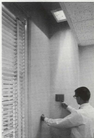
Device on sidewall controls supply voltage to infrared lamps in one zone.
