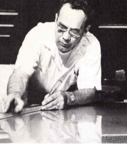
The stainless sheets marked up here for press work, were formed by the mechanical contractor, Temp-Control Corp., Portland.
