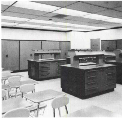
Concealed ducts in chemistry lab worktables carry exhaust from fume hoods down to mains installed beneath floor.
