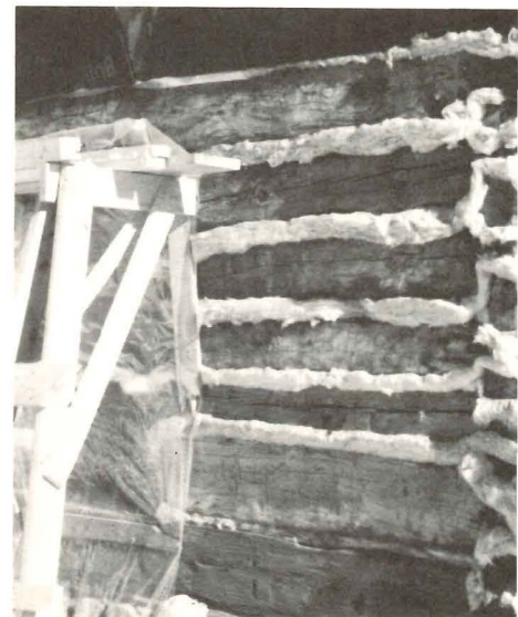
Old hand-shaped logs are chinked with fiberglass for the solar log house in Santa Fe's historic suburban district.
