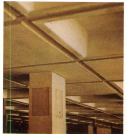
U of Tennessee Library, Chattanooga Architects: D. Derthick and Henley, Architects Contractor: H. E. Collins Contracting Co.
