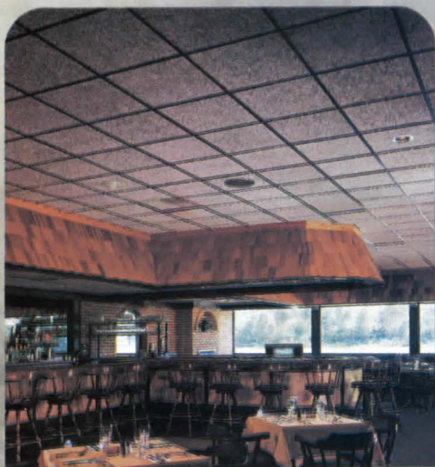
Shown above: frosted black. Acoustical Contractor: Northwest Acoustical, Inc., Southfield, MI
