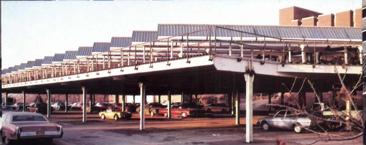
This 11,100 sq. ft. Sunpak installation is teaching Wagner College a lesson in economics — by making a dramatic reduction in fuel costs. Best of all, the sun is an energy source that won't run out. Ever.
