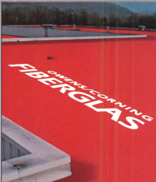
Single-layer FURI. Perma Ply No. 28 perf. base sheet. 2 plies Perma Ply-R. Gravel surface.
