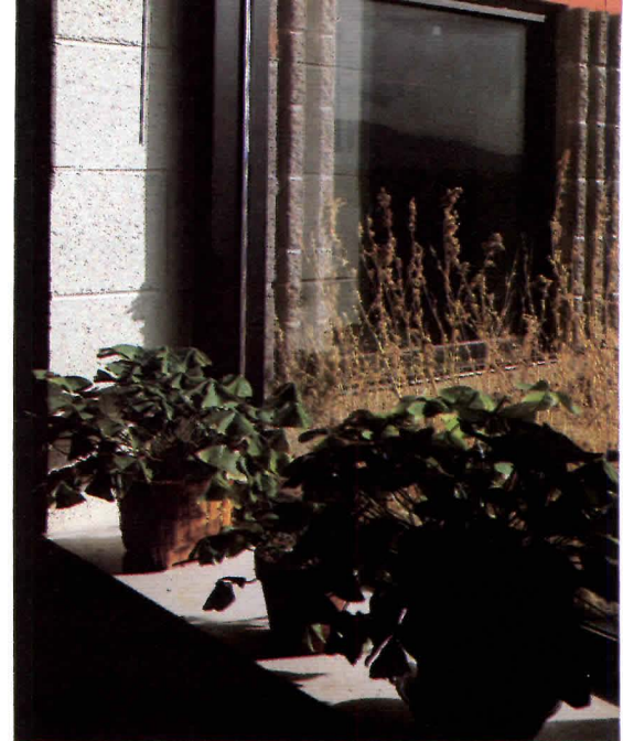
View from the interior, looking out, showing the extensive use of concrete masonry for passive solar heating and cooling and structural purposes.
