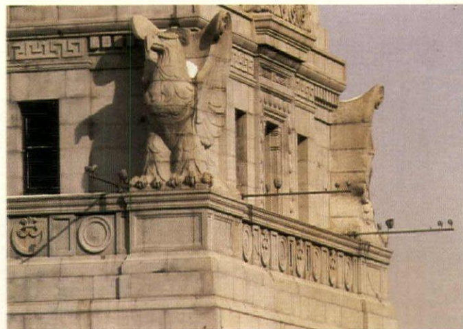
Galvanized pipe booms on the 20th floor hold precisely focused PAR fixtures to light the clockfaces and decorative stone features.
