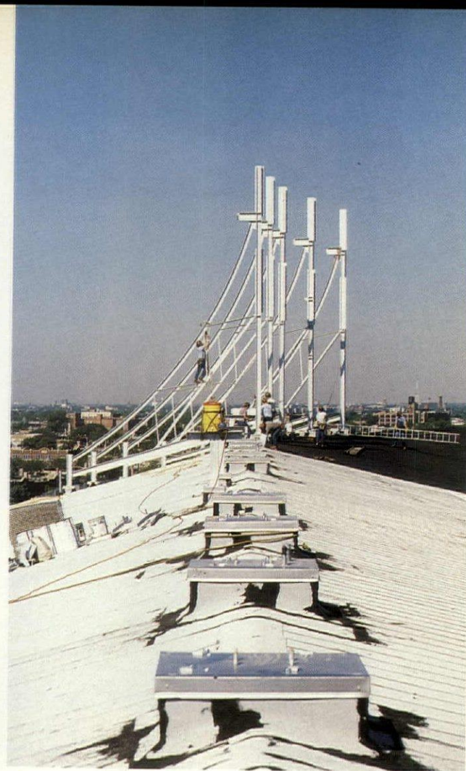
and curved braces. The reach was too long for a crane, even if there had been a suitable place to put one. So, everything on the stadium roof was put up with helicopters.
