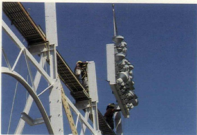
The racks that go between the columns and support the fixtures were prefabricated. The fixtures were mounted and the conduit installed before each rack was put into its frame. Catwalks link the light banks, not only to make service easy, but also for rooftop safety in the Windy City.
