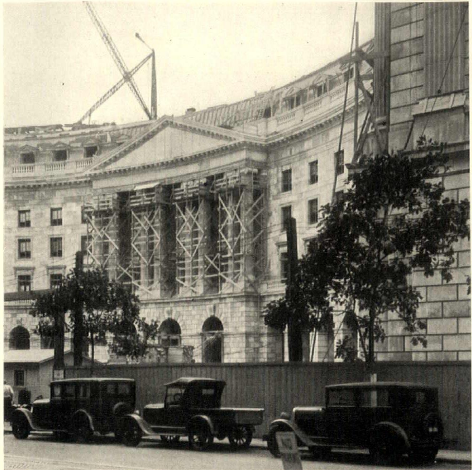
A recent progress photograph showing the central curved wall on the east elevation of the Post Office Building
