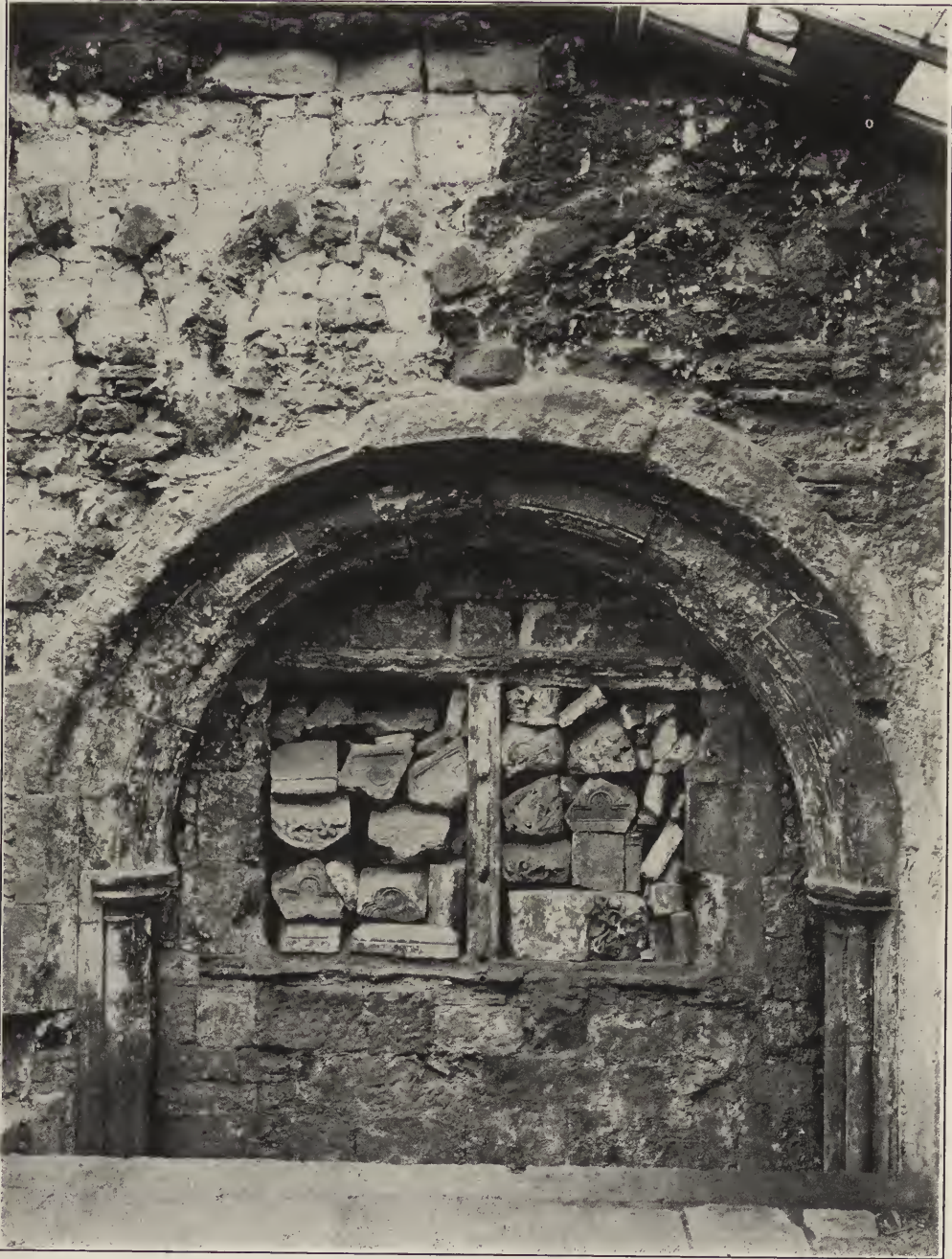
THE REMAINS OF THE ELEVENTH CENTURY ST. CATHERINE'S CHAPEL, THE CHAPEL OF THE MONASTIC INFIRMARY, SHOWING THE FEW ARCHES OF TRUE NORMAN TYPE THAT REMAIN.
