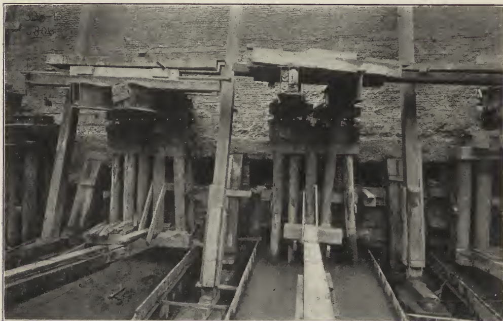
METHOD OF SHORING ADJOINING BUILDING FOR FOUNDATION OF ROYAL QUEEN BUILDING, NEW YORK.
