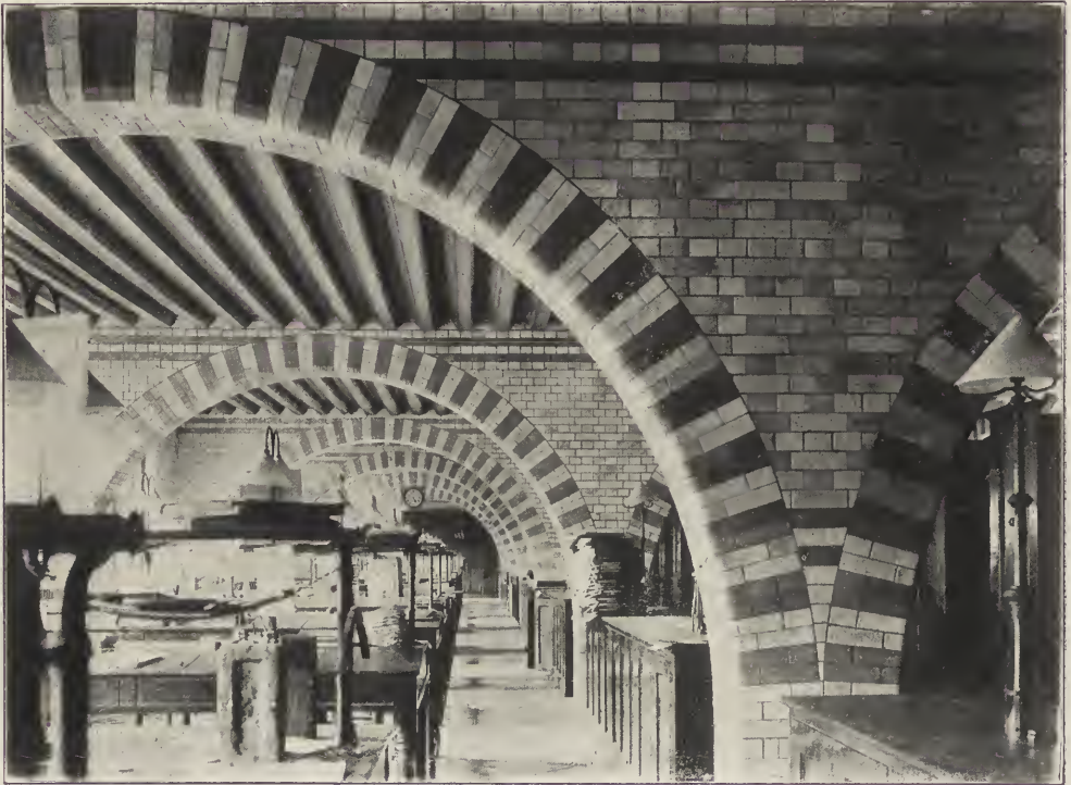
VIEW IN THE NORTH BLOCK, SHOWING A CONCRETE FLOOR CARRIED ON "IRON DECKING"—PRUDENTIAL ASSURANCE COMPANY'S BUILDING.
