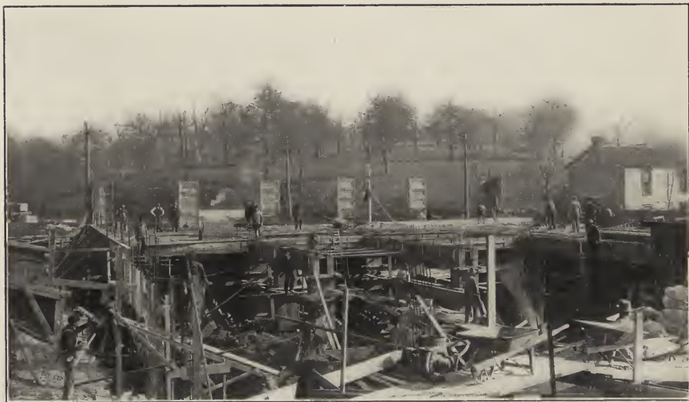
VIEW OF FOUNDATION, SHOWING THE GROUND FLOOR GIRDER FORMS AND STEEL REINFORCING RODS PROTRUDING FROM THE BOXES—TERMINAL WAREHOUSE.
