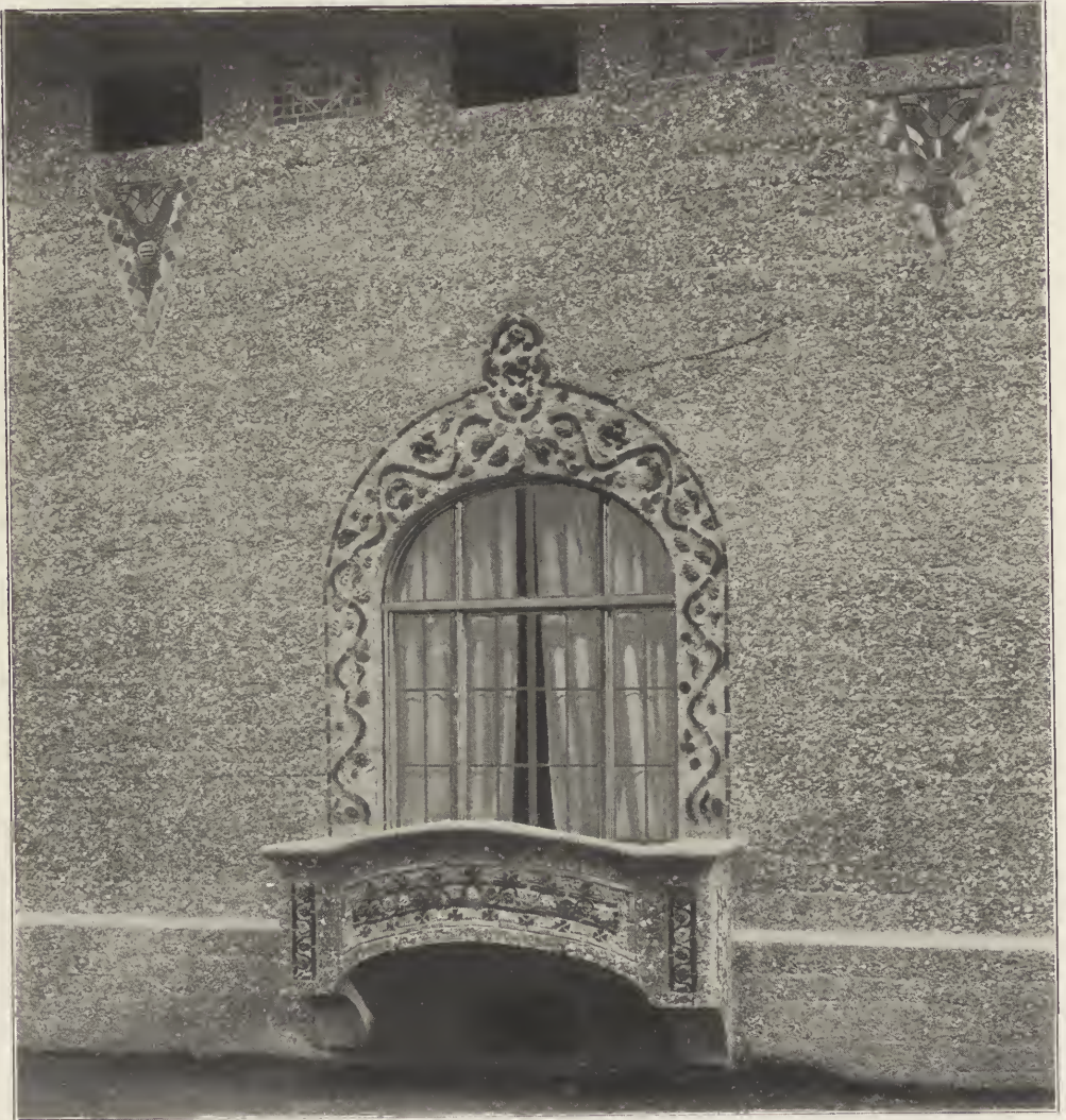
DETAIL OF REINFORCED CONCRETE RESIDENCE AT SOUTH ORANGE, N. J. (By courtesy of Vulcanite Cement Company.)
