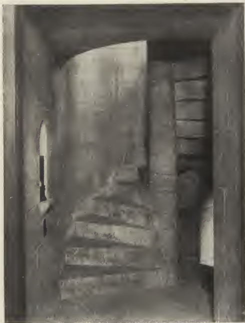
DETAIL OF THE SPIRAL STAIR IN THE NORTHWEST CORNER OF THE TOWER. ST. THOMAS' CHURCH. Cram, Goodhue & Ferguson, Architects.
