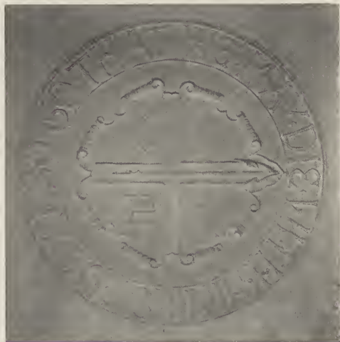
THE SEAL OF ST. THOMAS, EXECUTED IN PLASTER ON THE CEILING OF THE SACRISTY. ST. THOMAS' CHURCH, NEW YORK CITY. Cram, Goodhue & Ferguson, Architects.
