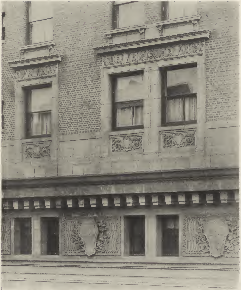
DETAIL—STRING COURSE, PANELS AND FIFTH FLOOR WINDOWS, HOTEL BILTMORE, NEW YORK CITY.
