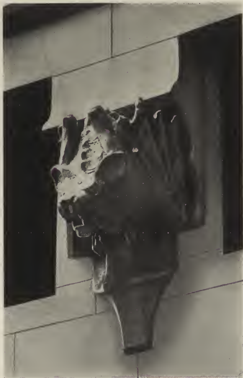
DETAIL—A GARGOYLE FROM THE WOOLWORTH BUILDING, NEW YORK CITY. Cass Gilbert, Architect.
