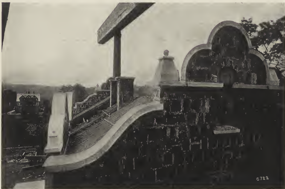
PROGRESS PHOTOGRAPH SHOWING "MISSION" GABLE END, BEFORE STUCCO WAS APPLIED, "GRAMATAN COURT," BRONXVILLE, N. Y.
