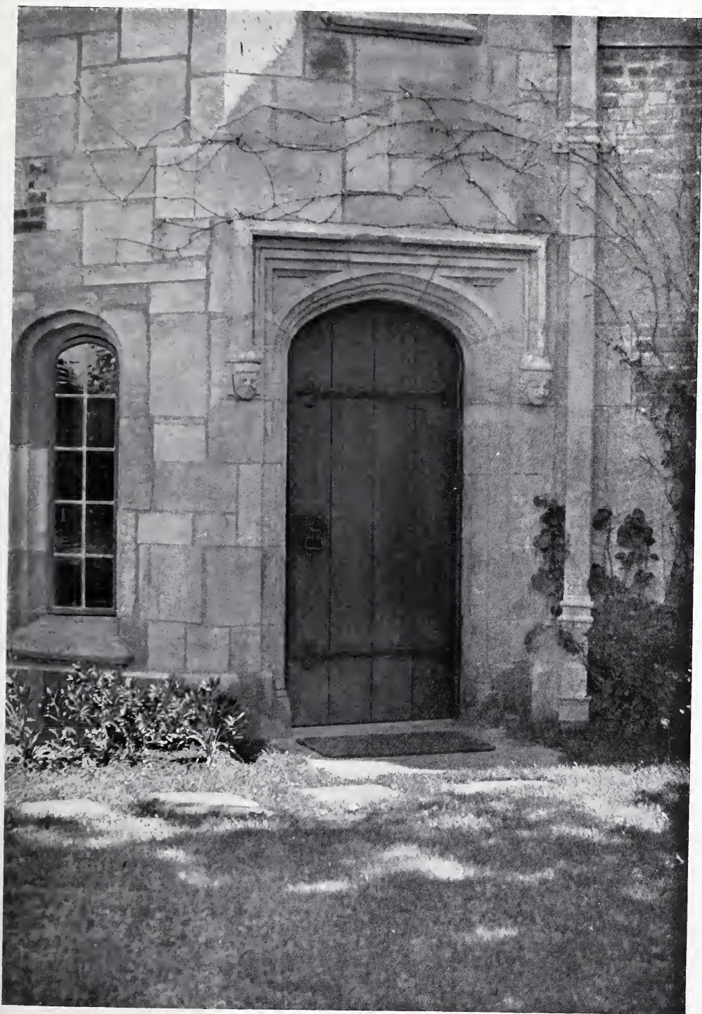
DOORWAY IN SMALL STAIR TOWER—RESIDENCE OF STUART DUNCAN, ESQ., NEWPORT, R. I. JOHN RUSSELL POPE, ARCHITECT.
