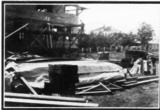
Sisalkraft used to cover materials. This same Sisalkraft was used over the sheathing in place of building paper
