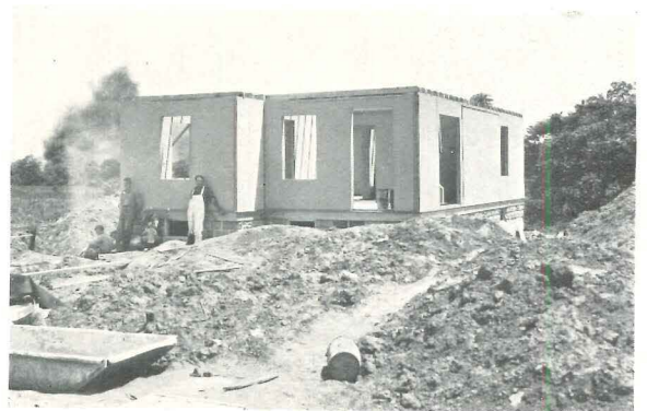
And 4 hours labor sees all partitions up, job ready for roof framing with pre-cut rafters.
