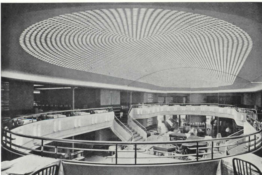
Fig. 8. In this cafe in Paris, architect Roux-Spitz has achieved a thin and shallow translucent dome by means of a system, poured in place and similar to Fig. 1.
