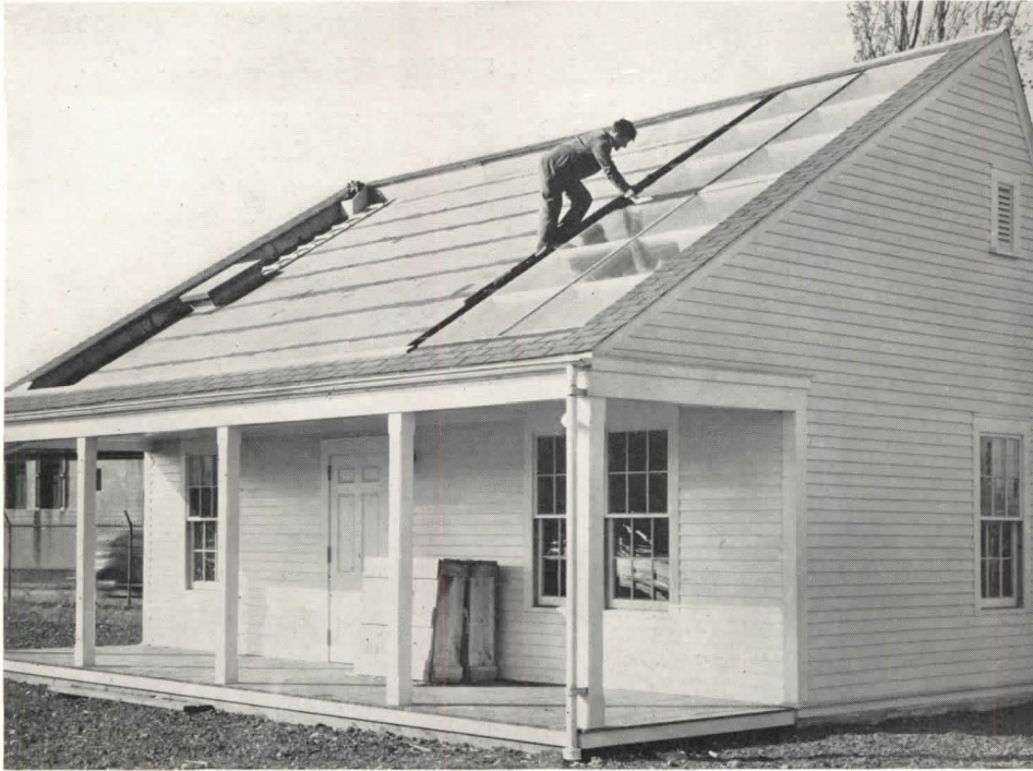
"Heat trap" in the roof of M.I.T.'s new experiment in conversion of solar energy. Note (upper left) the pyrheliometer, an instrument for recording sunlight intensities.
