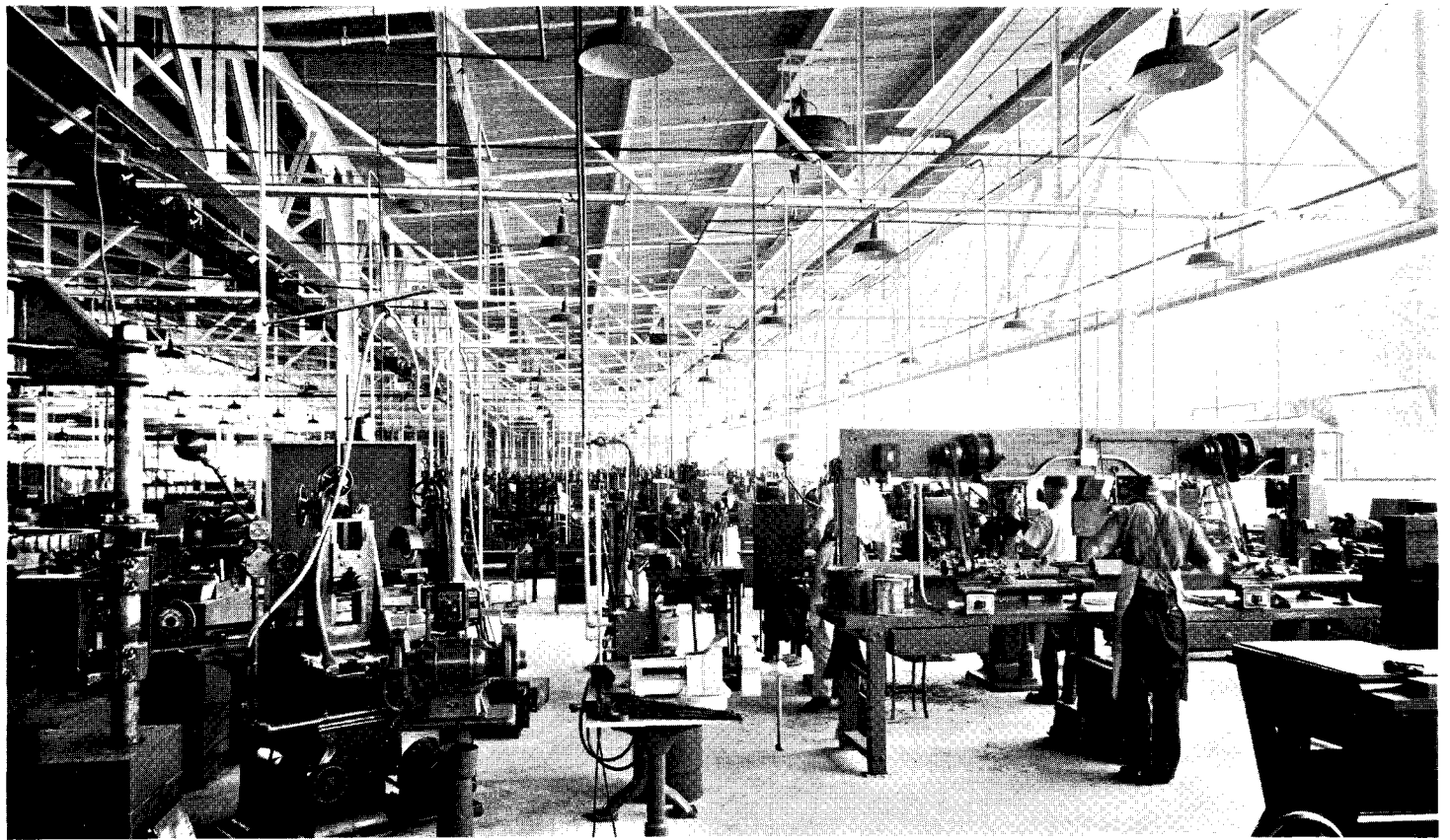
General manufacturing area: note new projection-type unit heaters and bus-duct power distribution.
